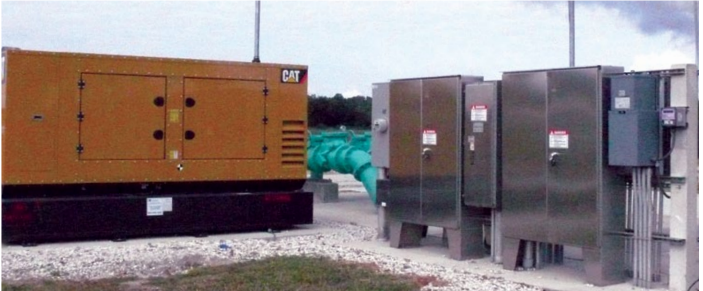
Polk County's waste water pump stations can be controlled with the help of AlarmAgent.com's web-based monitoring, alarm notification and control system.
